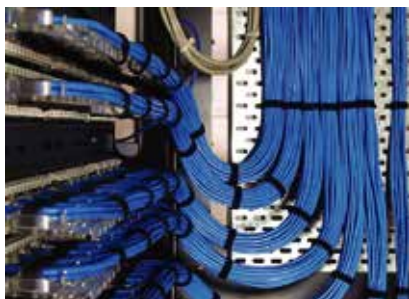
Structured cabling & Networking
